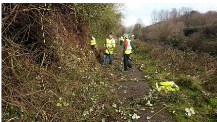
Photo: IWA West Country Branch Work Party at Lyndale Avenue, Bridgwater & Taunton Canal (photo by Mike Slade)
