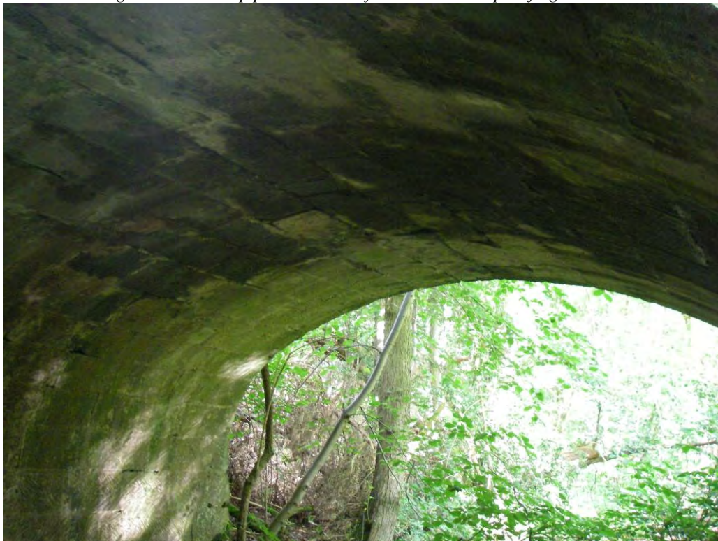
Plate B.2: Bridge arch has damp patches due to failed deck waterproofing
