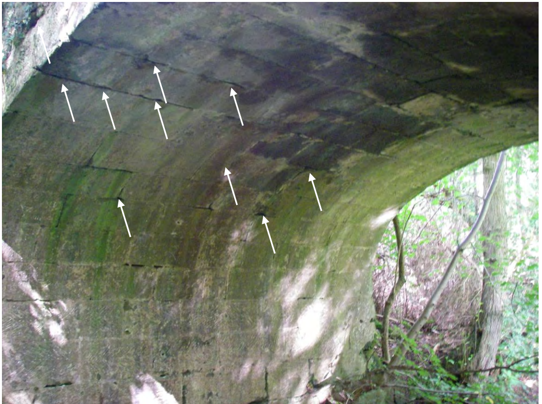
Plate B.3: Drier areas of bridge arch showing missing mortar joints
