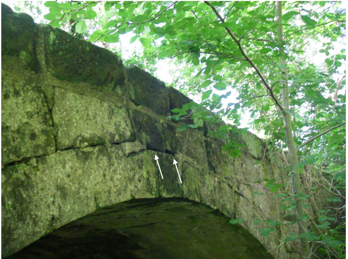
Plate B.4: Example of crevices in elevations
