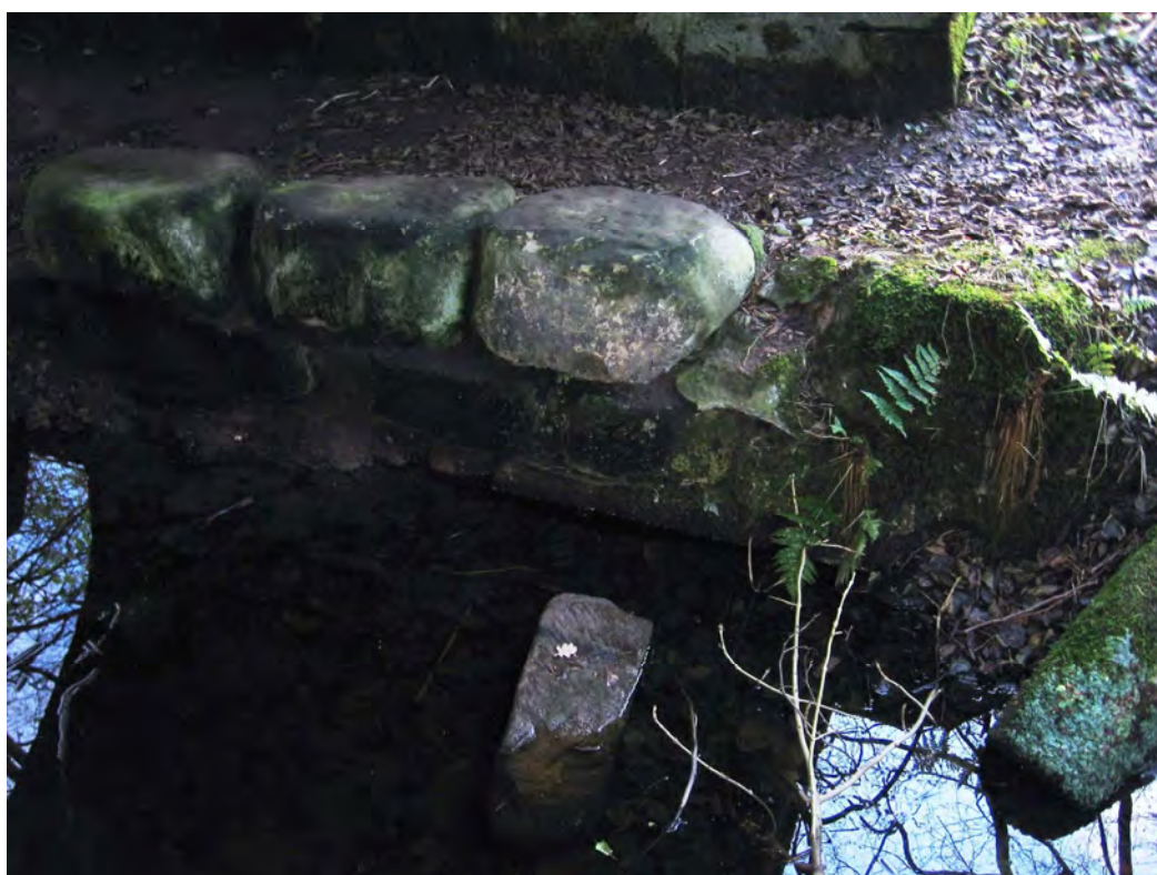
Photo(18): South towpath support wall in poor condition.
