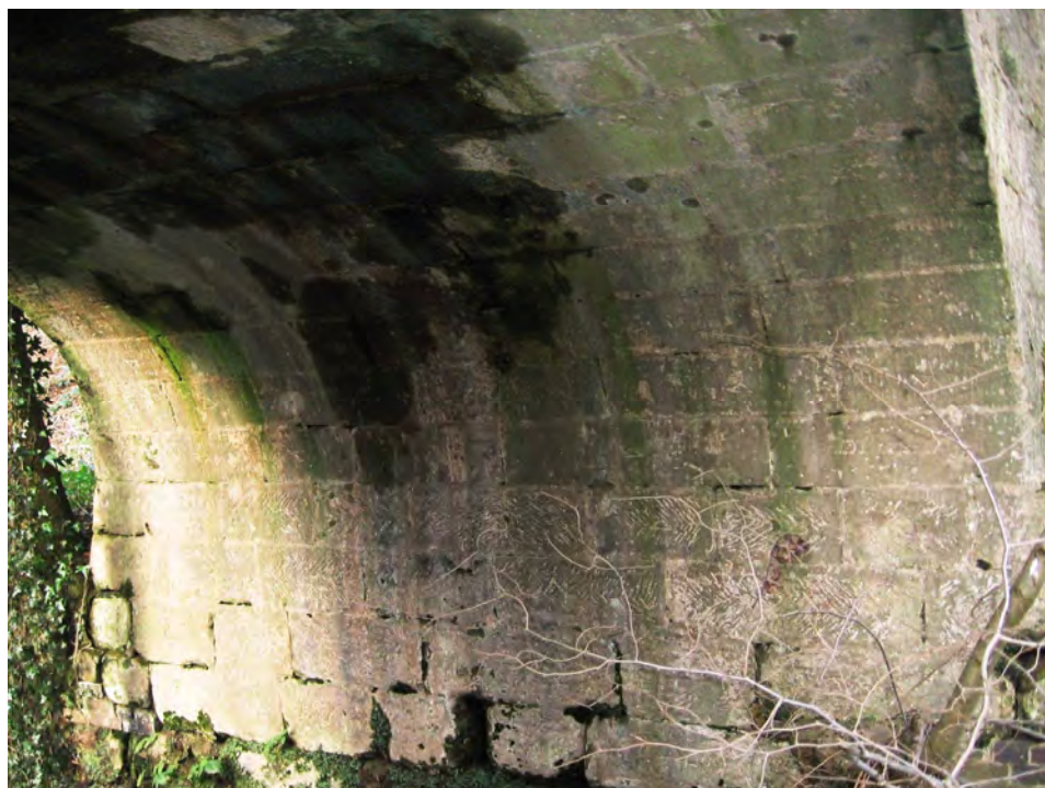
Photo(15): North abutment and arch ring, note water penetration to apex of arch.
