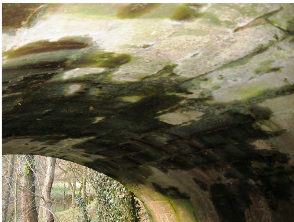
Photo(16): Arch barrel apex in fair condition, except for extensive water penetration.
