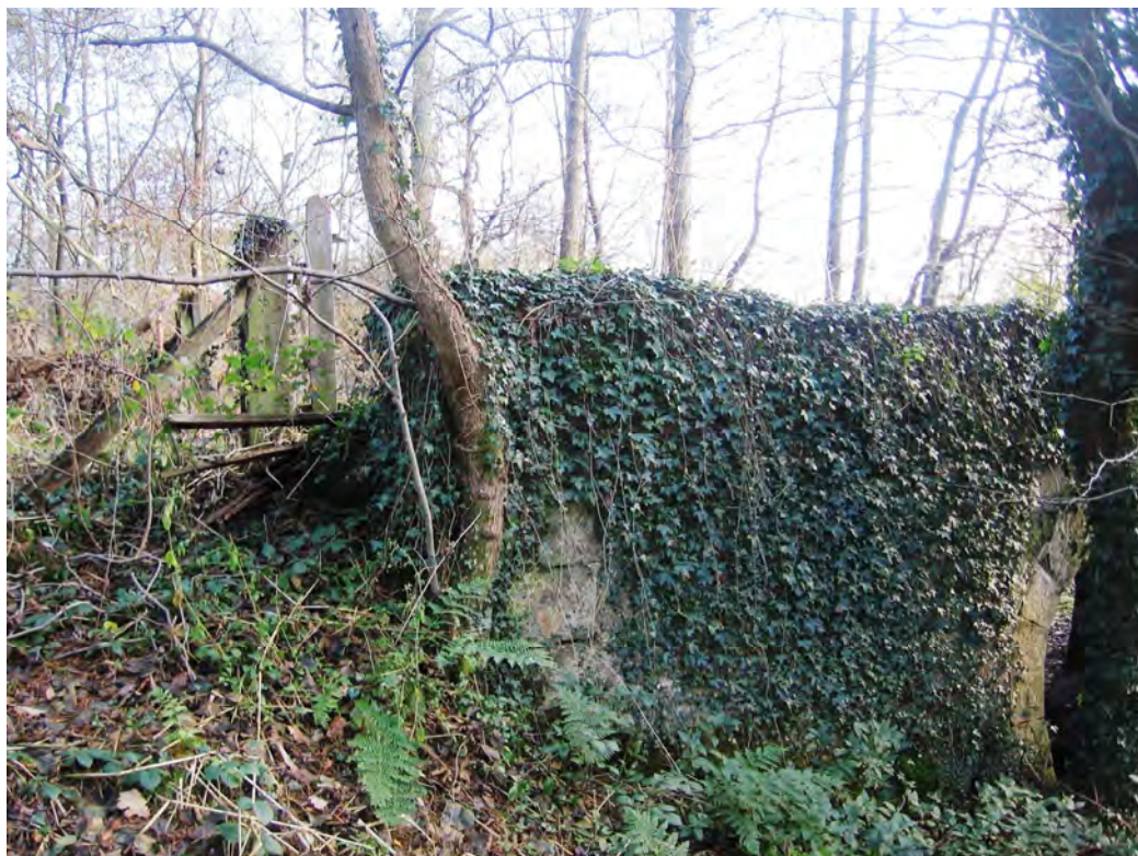
Photo(21): West elevation, north spandrel heavily overgrown with Ivy.
