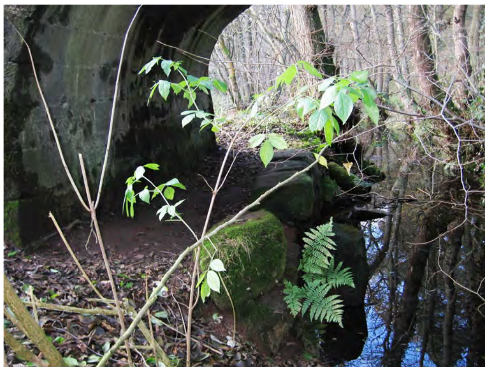
Photo(14): South abutment viewed from east elevation, towpath in poor condition.
