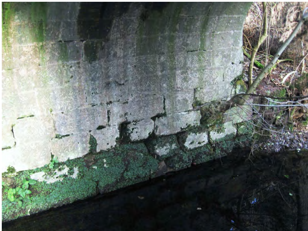
Photo(17): North Abutment from West elevation in poor condition.
