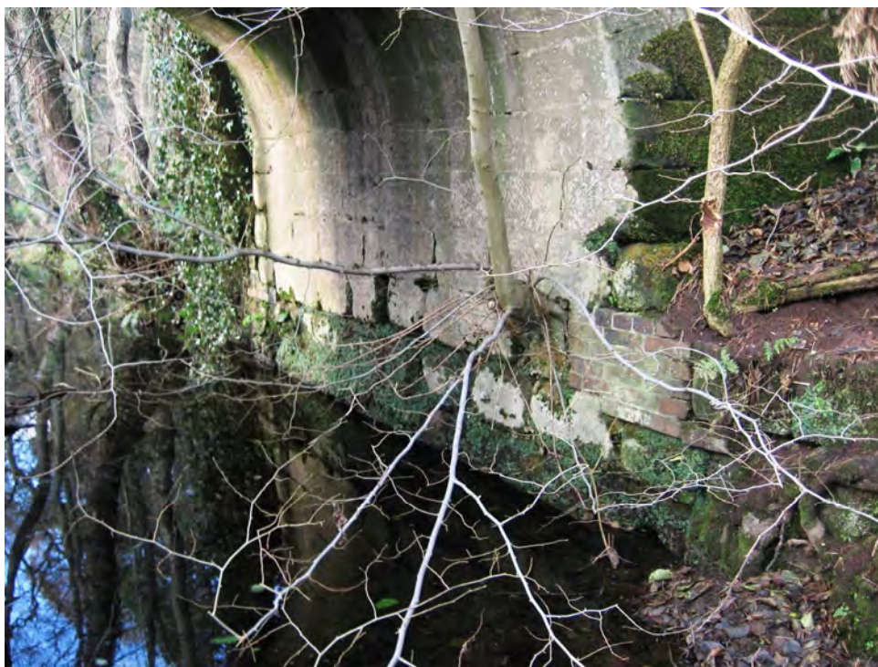
Photo(13): North abutment viewed from east elevation in poor condition.
