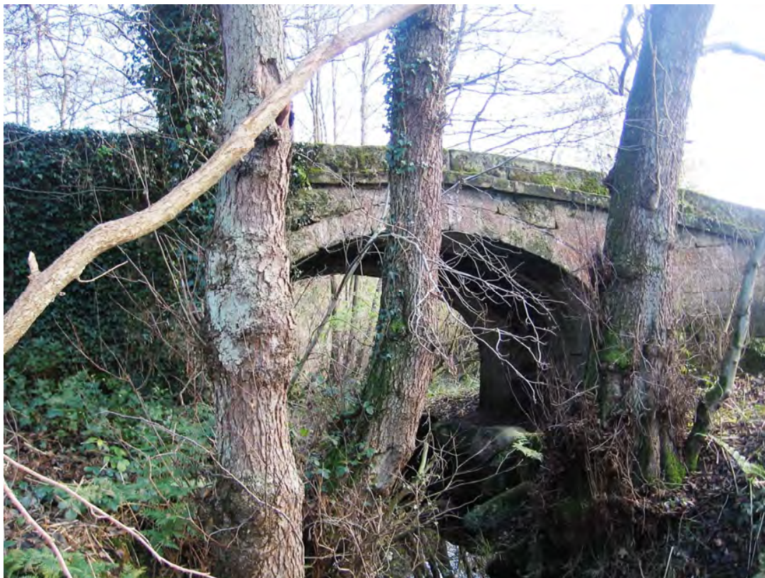
Photo(19): West elevation, heavily overgrown with trees and vegetation.
