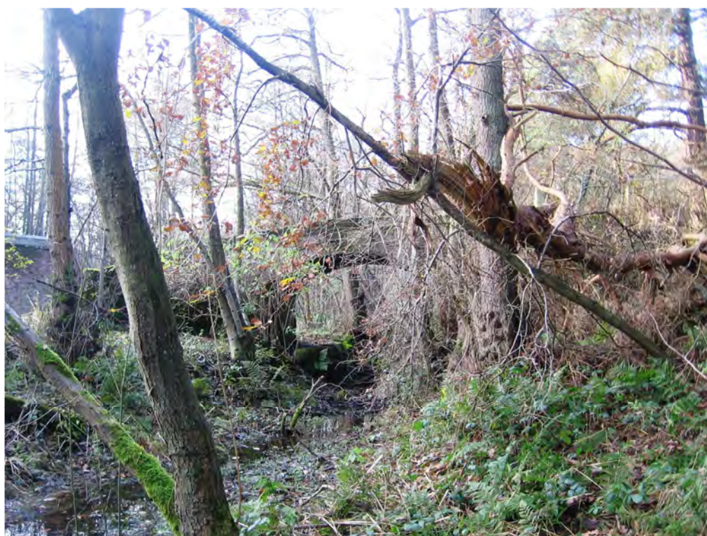
Photo(8): East elevation of seventy bridge heavily overgrown.
