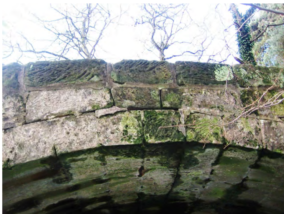
Photo(10): East elevation, apex stone of arch ring settled denoted by gap.
