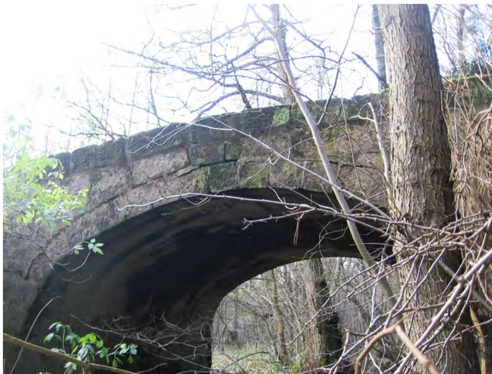
Photo(9): East elevation, showing arch ring separation.
